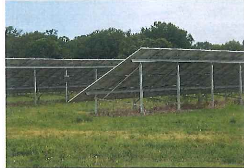
Example of a Solar Conversion System, Ground-mounted
