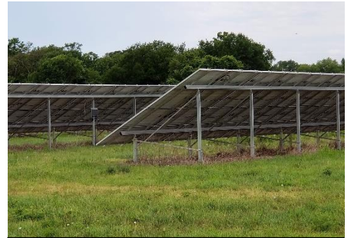
Example of a Solar Conversion System, Ground-mounted
